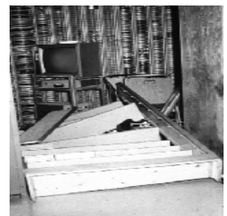
Example of earthquake damage.
